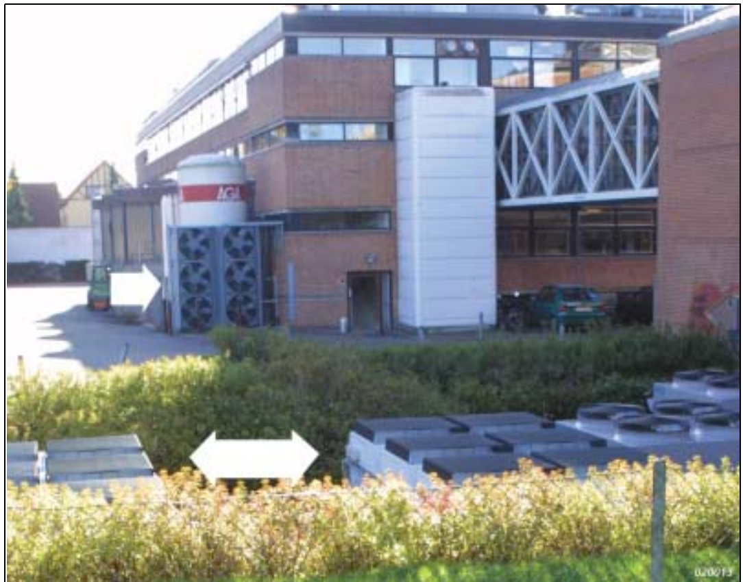
Fig. 1 Chemical plant with horizontal (close to fence) and vertical (on building) arrays of cooling fans
